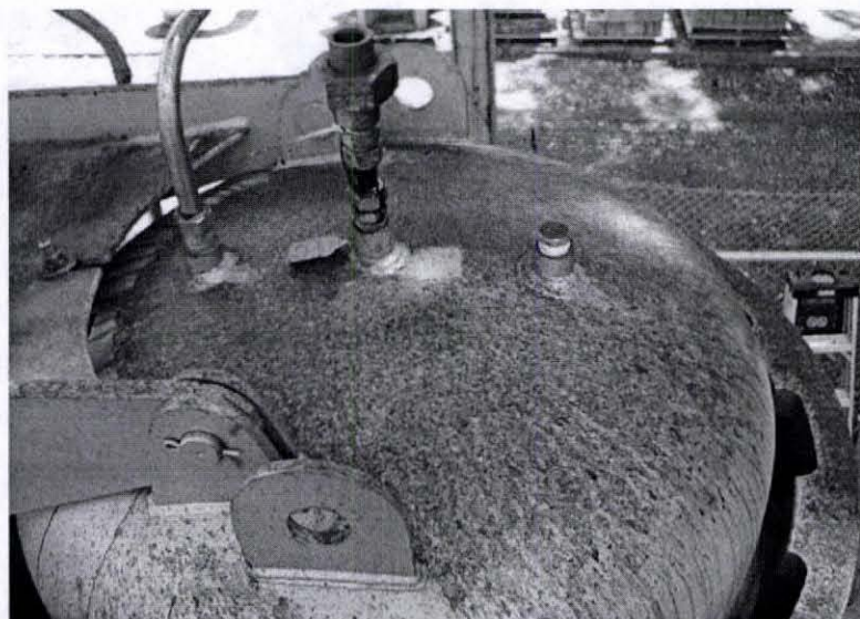
Figure 7.3 Following the burst of the rupture disk mounted on the top of the demonstration reactor (housed in the hexagonal casing), a plume of smoke and a shower of tarry vapors vented quickly, resulting in the dark stain shown in this photograph.
