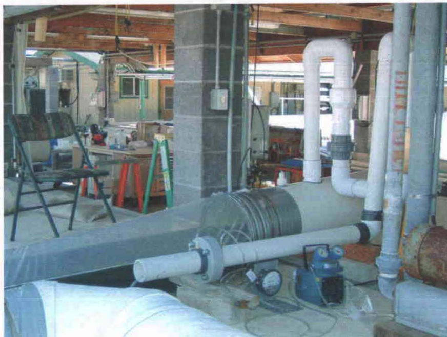
Figure A.5. Photograph showing the gas sampling system and the orifice meter attached to the photobioreactor vent at Mera Pharmaceuticals' facility.
