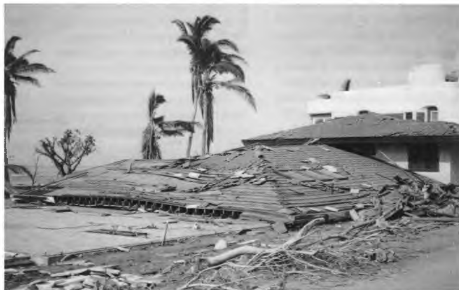
One of many homes on Kauai leveled by Hurricane Iniki. Photo by Ron Iwamoto, Richard Sato & Associates.
