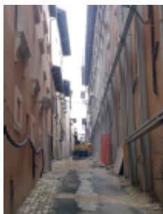
Figure 2. Reconstruction continues in L'Aquila, Italy. A side street off the main thoroughfare. Buttressing on the buildings on the right-hand side of the alley. Credit: Julie Dugdale, October 2019.
