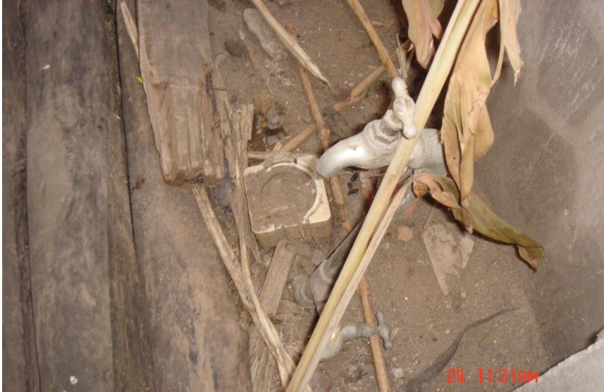
Picture 6.23 An Abandoned and Wasteful Water Meter
