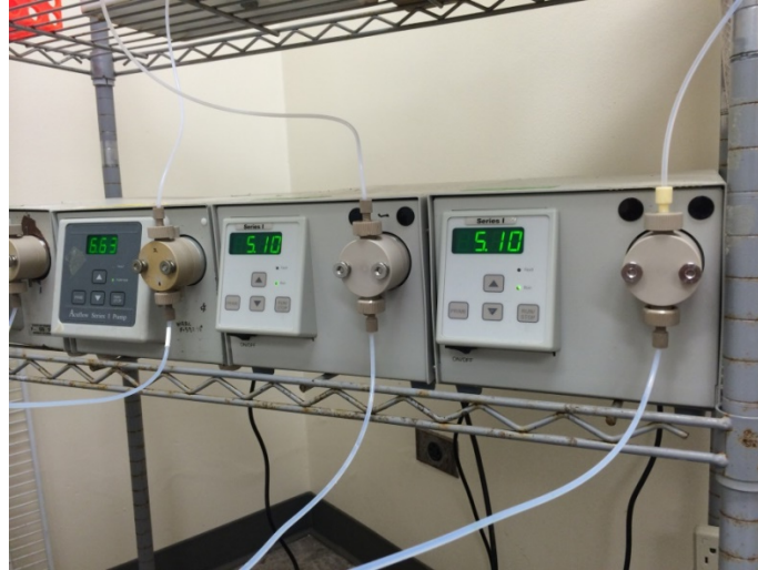
Figure 17: Liquid Metering Pumps
