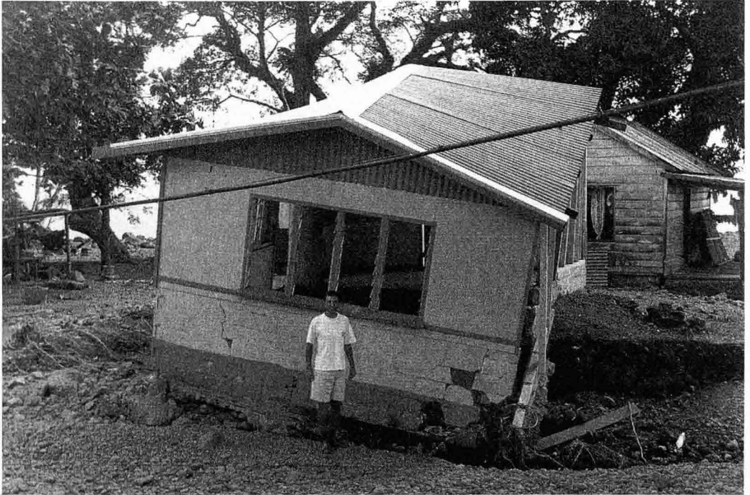
FIGURE 8. Property damage caused by stream floodwaters and erosion by coarse sediments on the island of Taveuni after Cyclone June.
