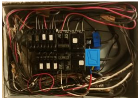
Figure B.4: Conventional household wiring retrofitted with non-intrusive high temporal resolution SEM
