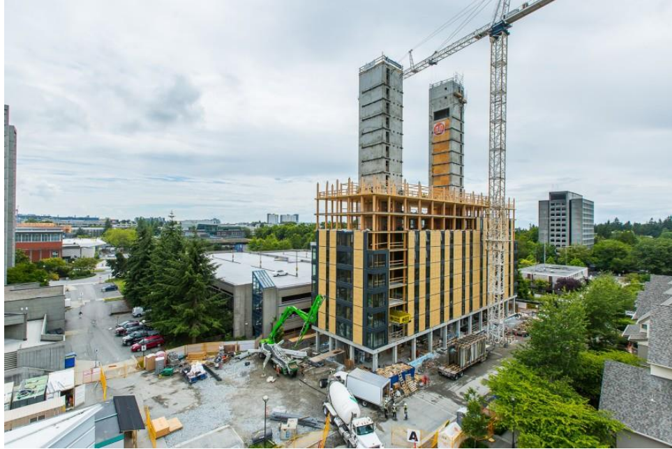
Figure 2.25: Brock Commons features two concrete stair cores and a hybrid wood-and-steel floor structure. by Acton Ostry Architects
