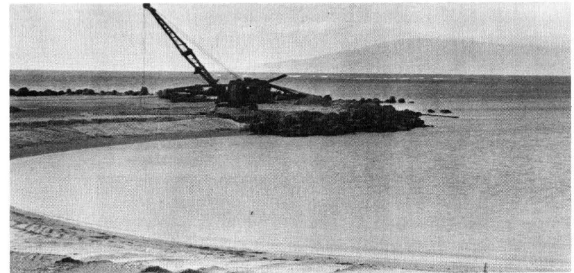
Pukoo is scheduled to be a site for a small resort development.
