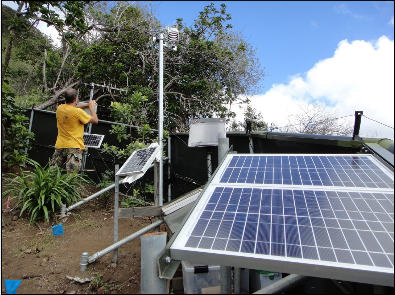
Figure 22. Remote Monitoring System Components
