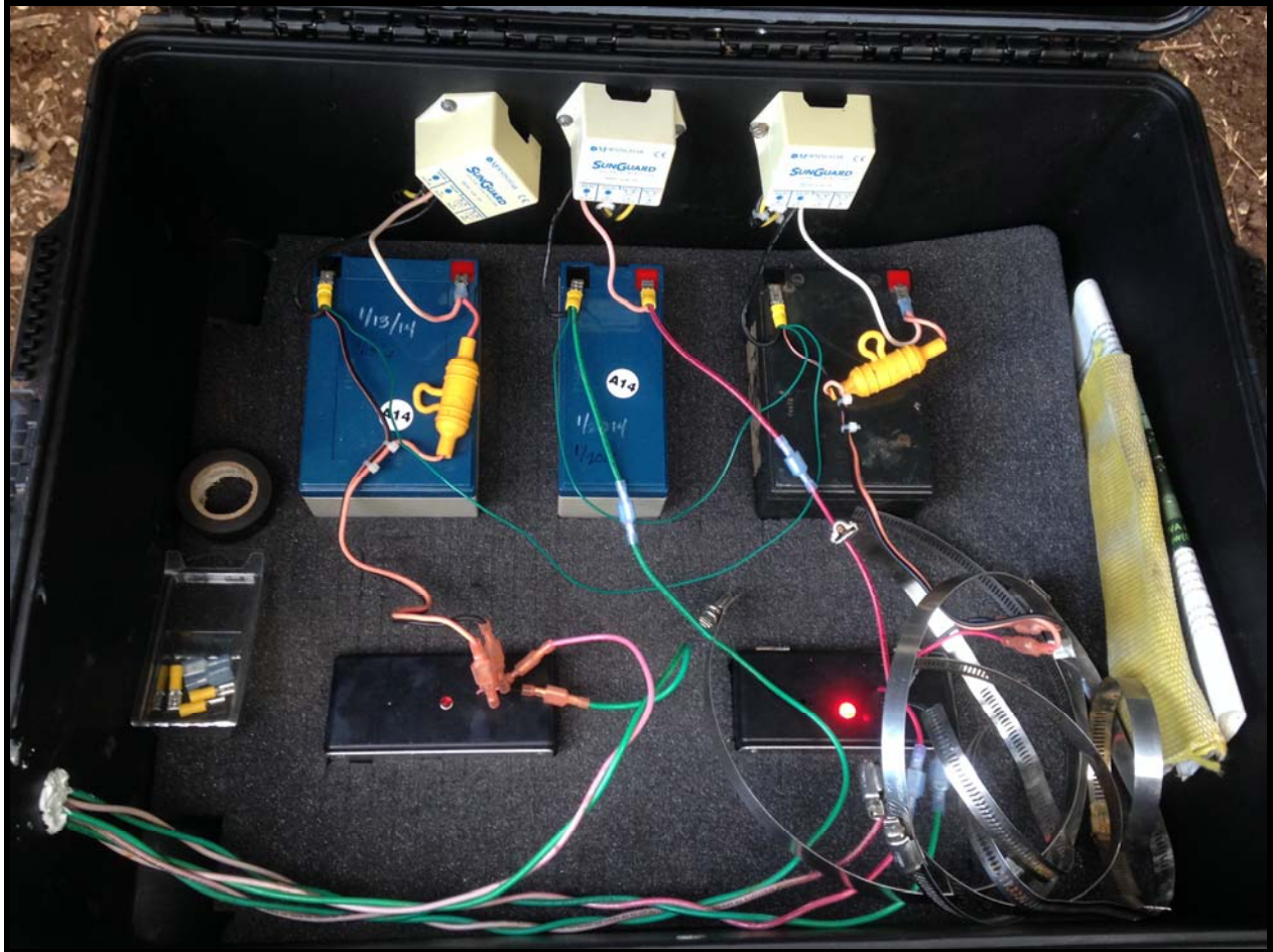
Figure 19. Weather proof housing used for electric components and batteries
