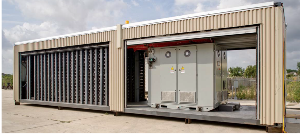
Figure 1.6. Xtreme Power's DPR™, a modular advanced lead-acid battery storage system [32]
