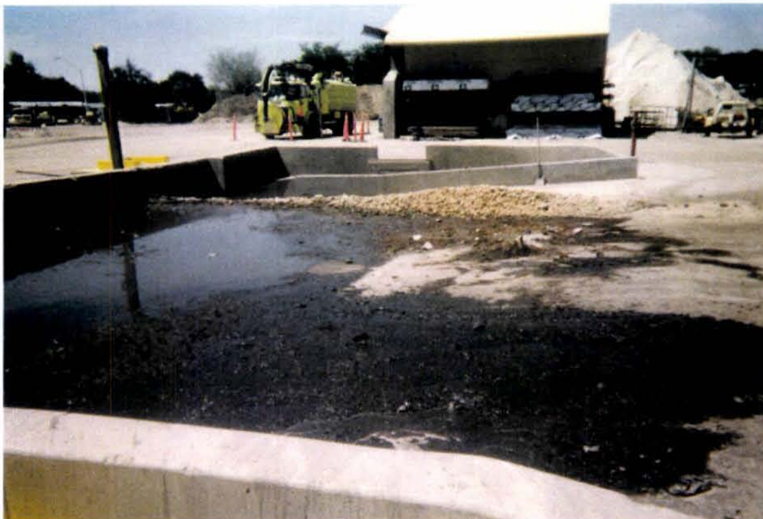
Figure 3.3 - Decant Basin at ACHD's Adams Street Facility (photo taken facing West)
