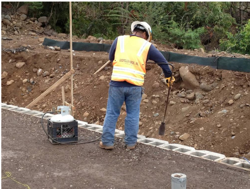
Figure 31 Geosynthetic Burned Through Using a Torch
