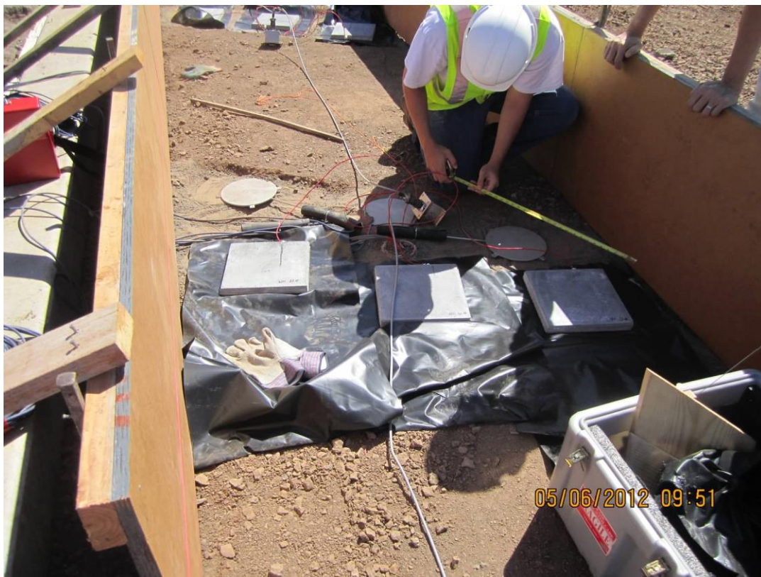
Figure 51 Nano Concrete Tiles Set Down on Plastic Sheeting Which Was Then Folded Over To Sandwich Them
