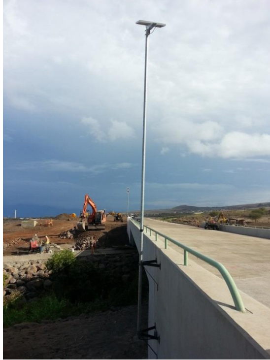
Figure 85 One 65 Watt Solar Panel at Abutment 2
