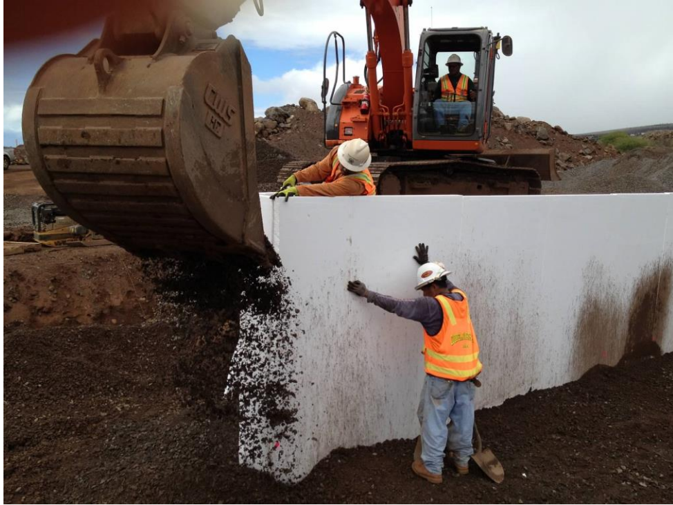
Figure 32 Styrofoam Placed in Front of Abutment 1 Prior to Placement of Rip Rap
