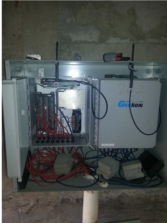
Figure 77 J-Box at Abutment 1 Containing the Wireless Transmitters (WT1 on left and WT2 on right)
