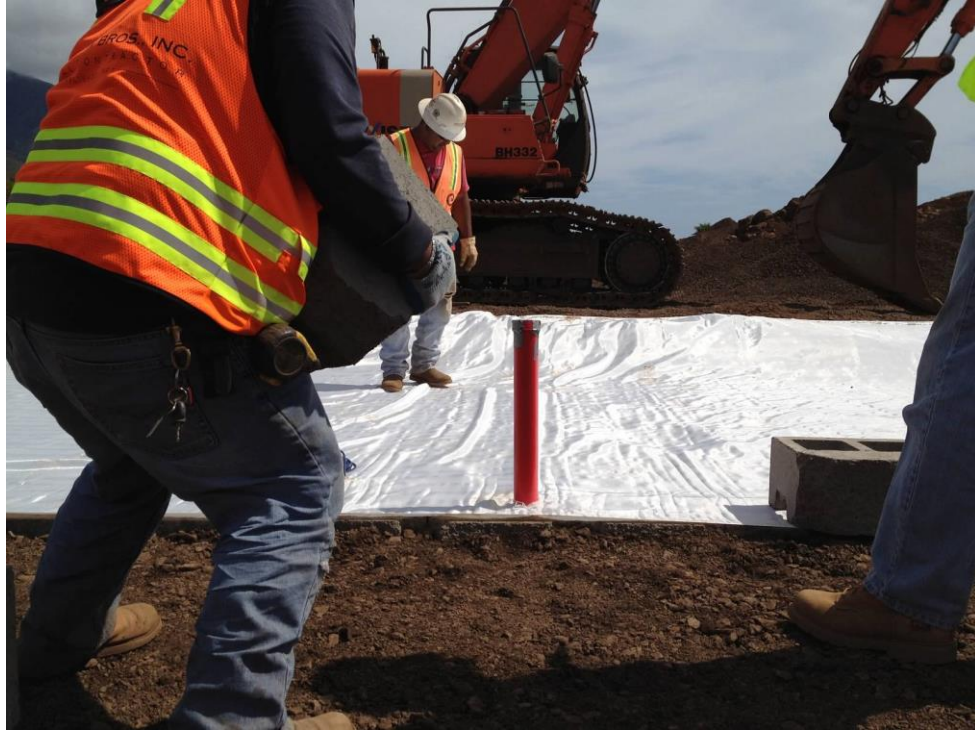
Figure 60 Inclinometer Casing Protruding Above Ground
