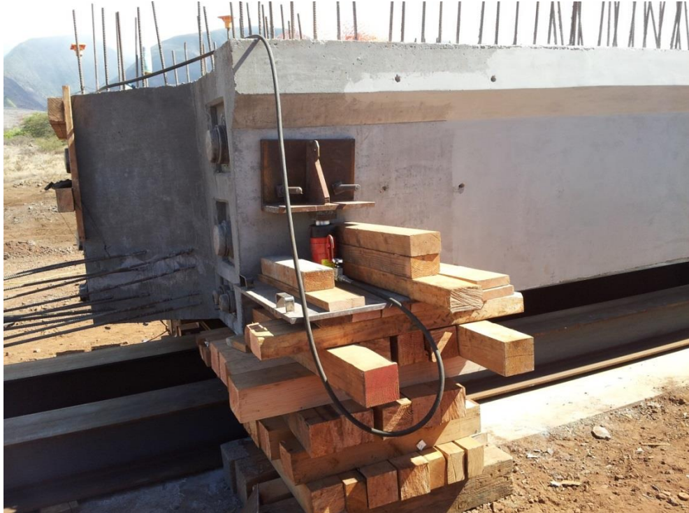
Figure 36 Hydraulic lift Raising the Tub Girder onto Two Steel Beams used as a Guide
