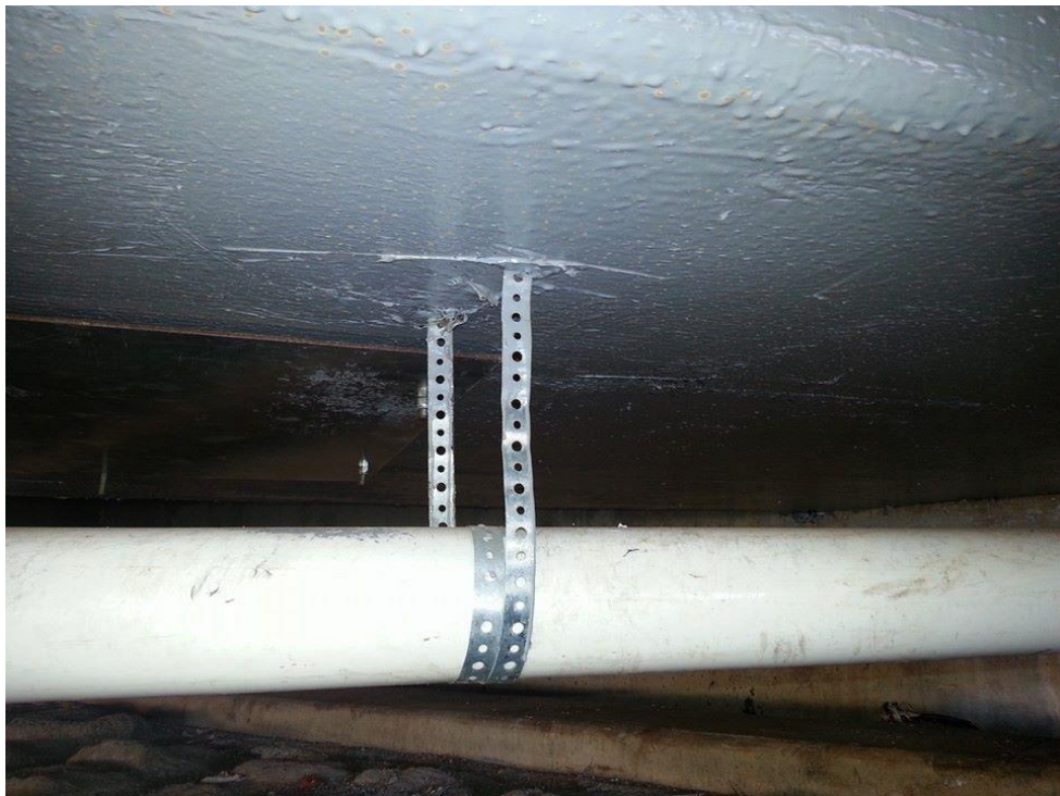
Figure 73 Steel Straps Used to Hold up PVC Pipes
