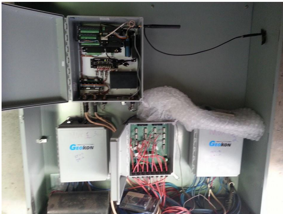
Figure 78 J-Box at Abutment 2 Containing the Three Multiplexers (Bottom Row) and One Datalogger (Top)
